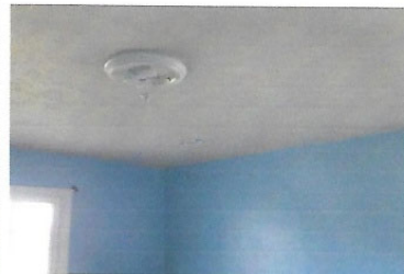
16-May-14 10:15 1234 E Main St, Anywhere ST 11111 Mark Shepard, photographer Test 3.1 - Main Flr NW Bedroom Ceiling
