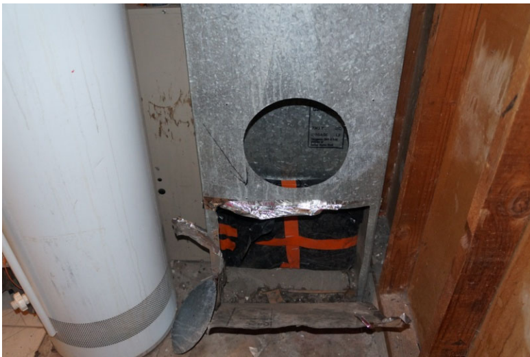
Non-AC unit Set Up
