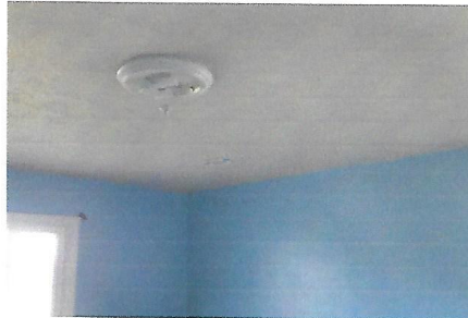
16-May-14 10:15 1234 E Main St, Anywhere ST 11111 Mark Shepard, photographer Test 3.1 - Main Flr NW Bedroom Ceiling
