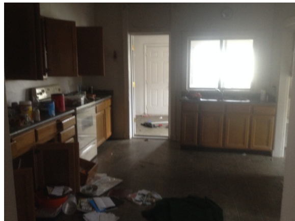
6-Mar-14 14:05 630 E Main St, Salt Lake City UT 12345 Mark Shepard, photographer Main Flr Kitchen
